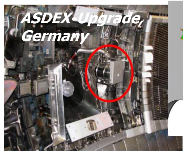
valve screened by a protecting tile
